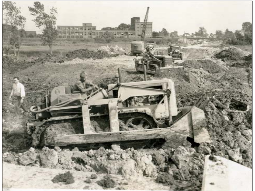
This 1939 image from the Thomas C. Wilson Photograph Collection shows construction on the Route 1 Bypass in Portsmouth.
